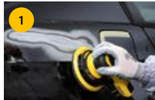
1 Remove paint on repair area, use net disc grit P80 or P120.
